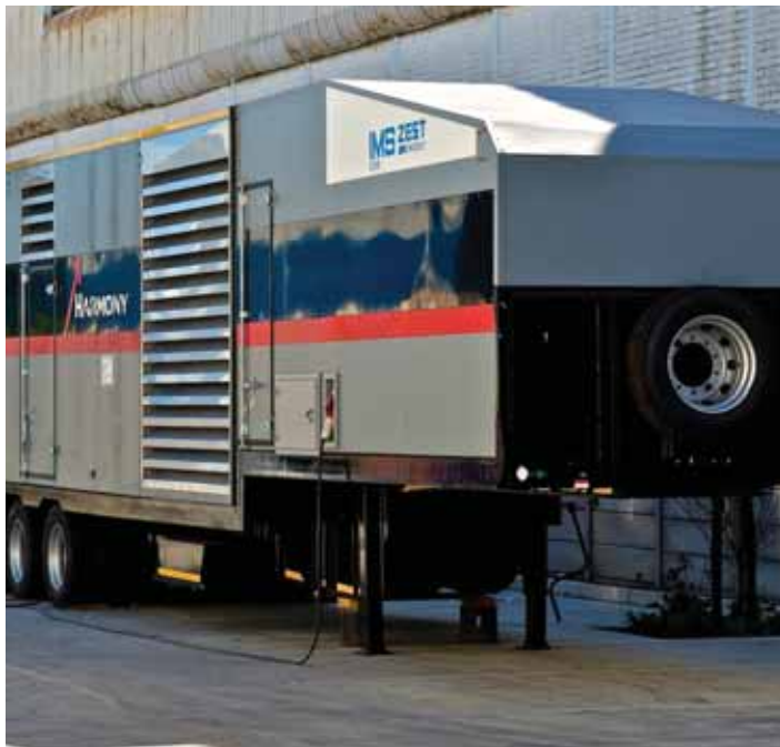
MOBILE DIESEL POWER GENERATION
